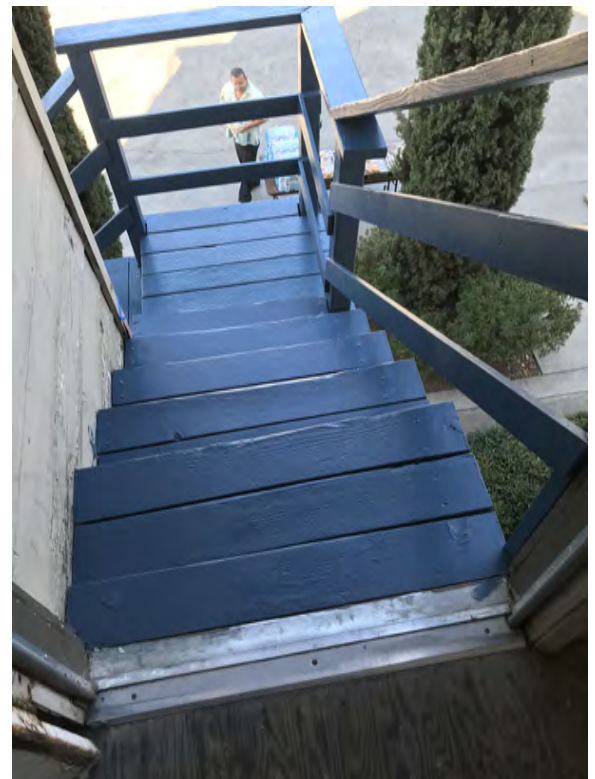
Concerns about primary, rear second floor stairs which are wooden
