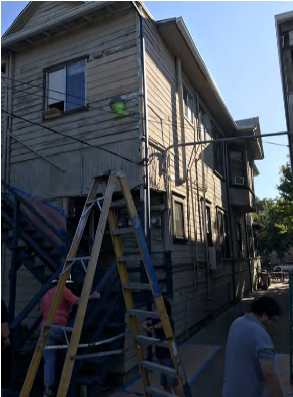
Concerns include exposed plumbing, building foundation settling, siding deterioration and single pane aluminum windows
