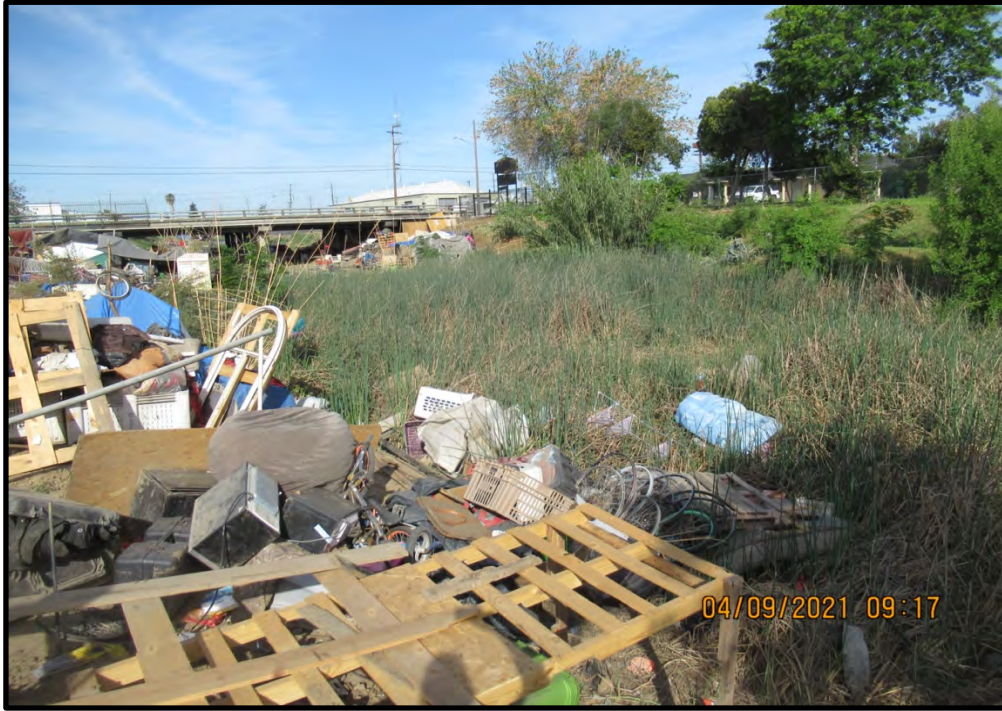
Trash and a patch of tules just downstream of the box culvert inlet area, looking northwest; 04/09/21. Water seeps around the north edge of the culvert inlet and ponds water in a low area upstream of the bridge.
