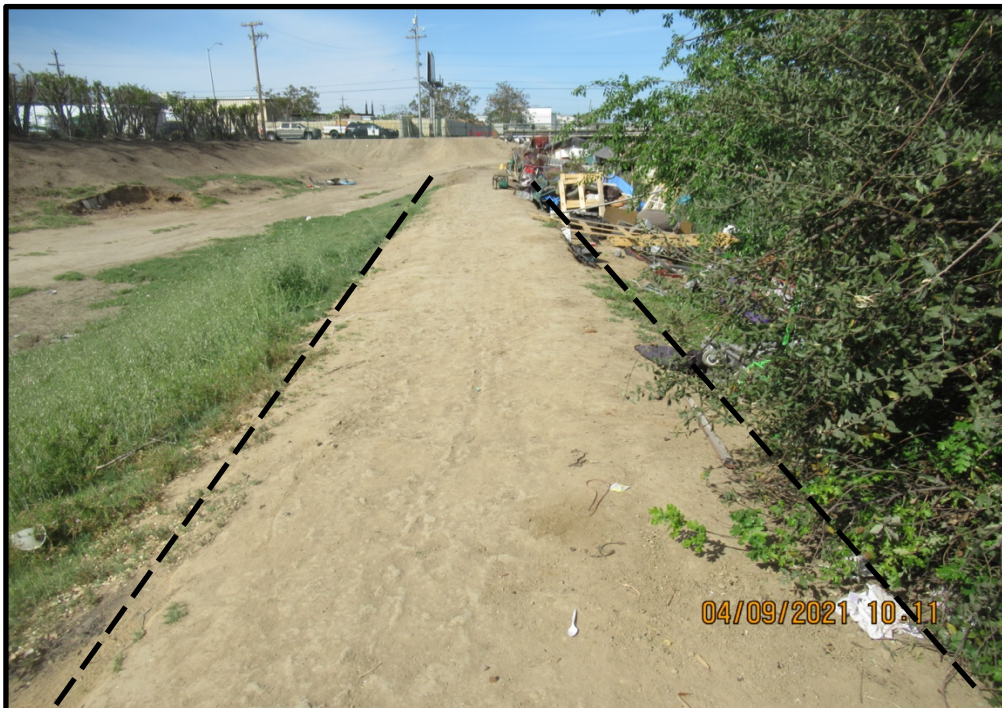
Top of the underground culvert system shown in the photo above, looking west from just downstream of the culvert inlet; 04/09/21.
