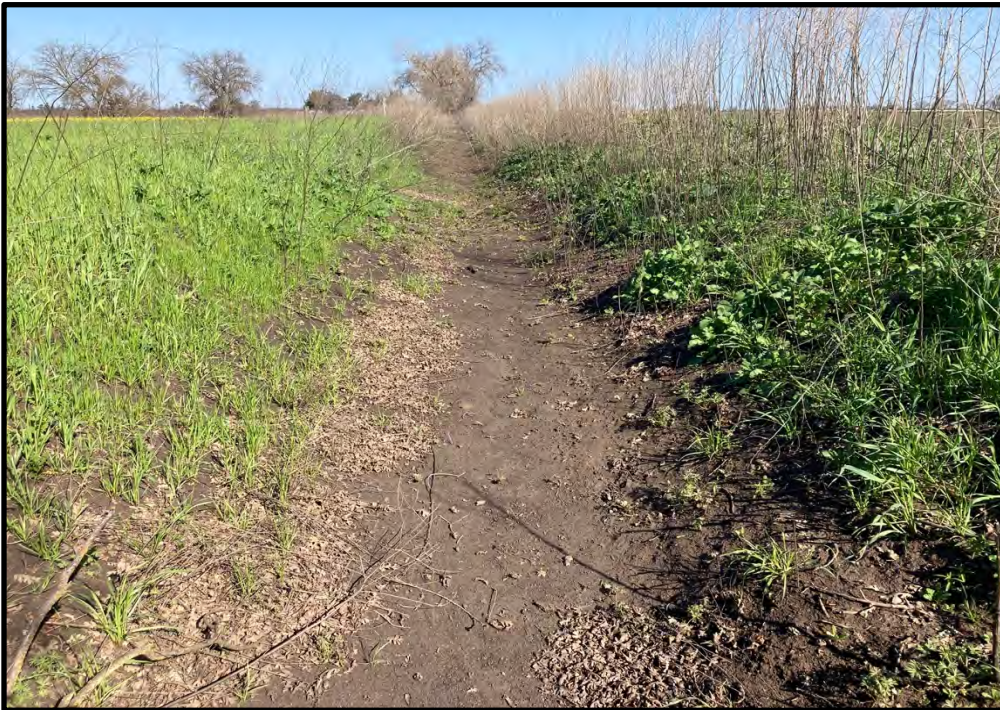
Constructed ditch along the west edge of the site, looking northwest from the southwest corner of the site; 03/16/23. Water in this ditch drains in to North Littlejohns Creek to the south of the site.
