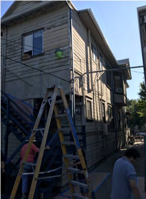
Concerns include exposed plumbing, building foundation settling, siding deterioration and single pane aluminum windows
