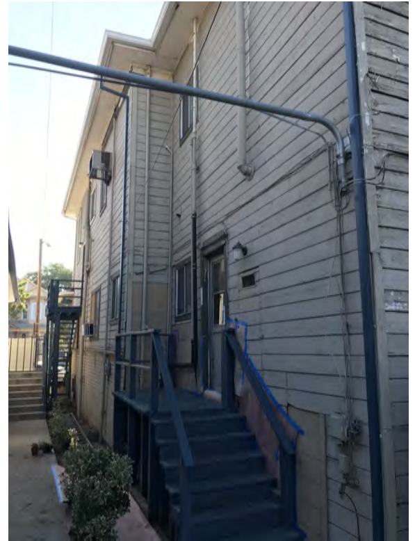
Concerns include wooden first floor exterior stairs, additional exposed plumbing Front, second story stairs are wood
